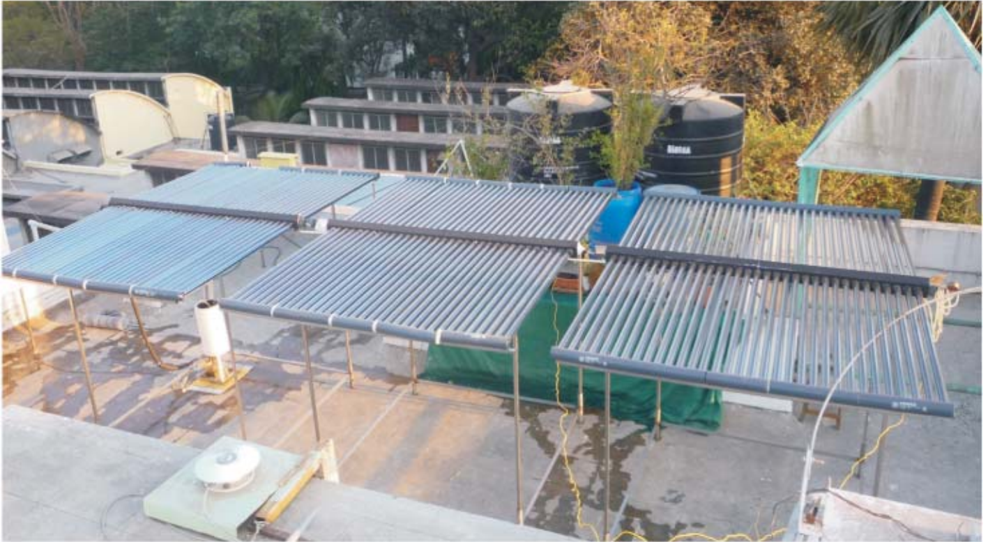
Figure 1: HP_SC Arrays Installed on HPL_IITB Terrace
